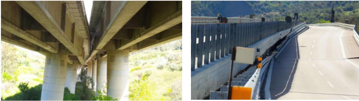
Figure 14. Flanking of the carriageways and state of the carriageway towards Catania of the “Himera” viaduct I” following the landslide of April 2015 (ANAS, 2016).
