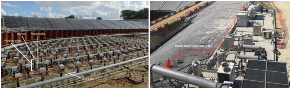
Figure 1. Haemers Technologies ISTD plant with Vapour Treatment Unit (VTU) (Gela site, 2018)
