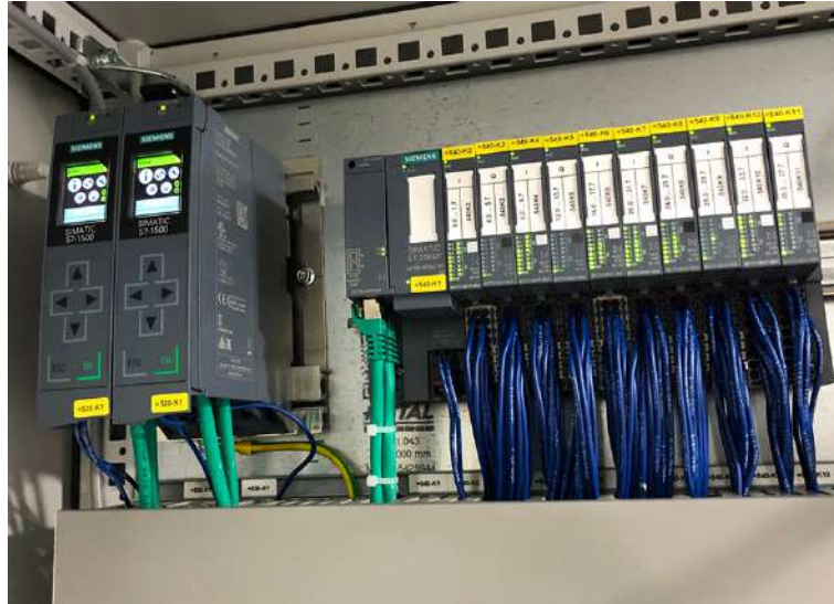
FIGURE 3.1: The electrical panel of a 4.0 machinery where is possible to see a Siemens S7 1500 PLC installed.
