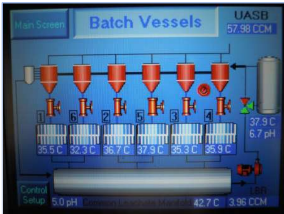
Figure 2.2.2. Control and setup panel
