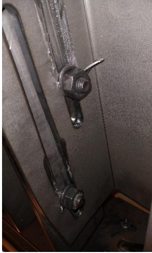
Figure 5.8. Scraping effect between bolt washers and edges of slotted holes
