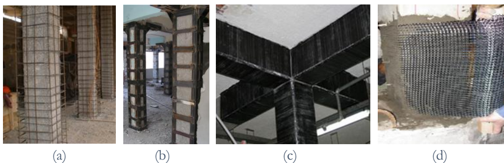
Figure 2.2. Jacketing techniques: (a) RC, (b) steel, (c) FRP and (d) TRM jacketing.
