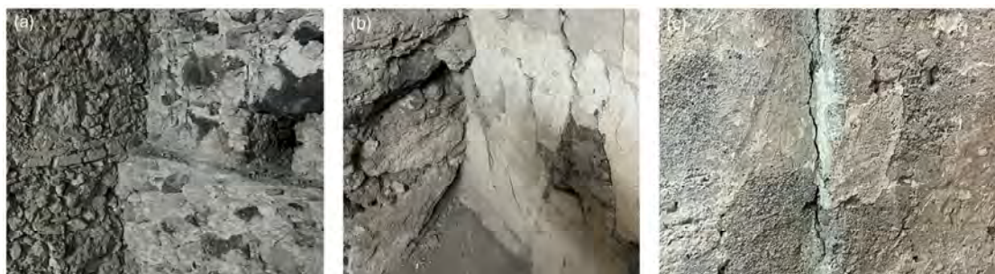
Figure 5. Three different examples of contact points between walls stratigraphic units: (a) USM 7 up USM 3; (b) USM 19 up USM 1; (c) USM 11 up USM 8.
