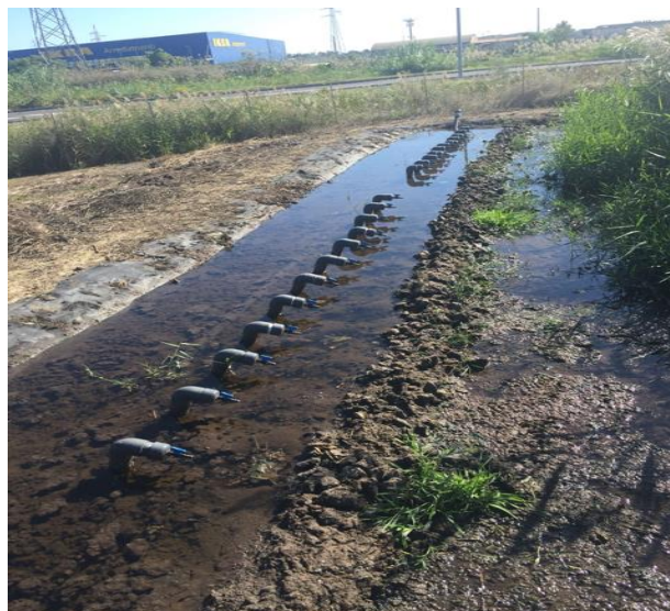
Figure 5.1: IKEA - New inlet system in HF bed
