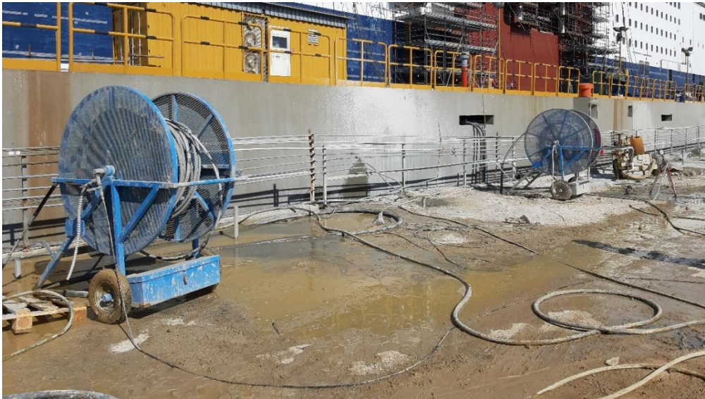
Figure 7-25: Injection system at Palermo Industrial Port.
