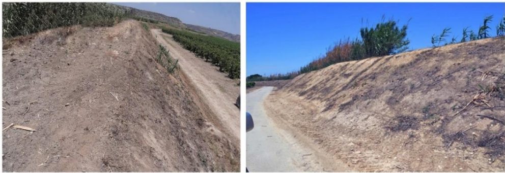
Figure 4-2: Current situation of Dirillo earth levees – field survey on the 2 nd July 2019.
