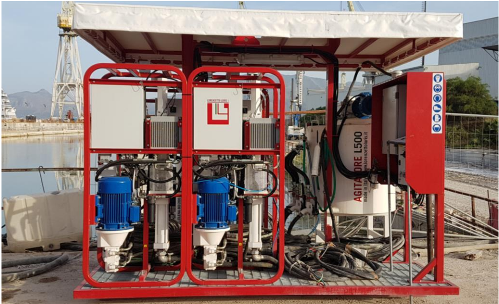
Figure 7-26: Pumping plant used at Palermo Industrial Port.
