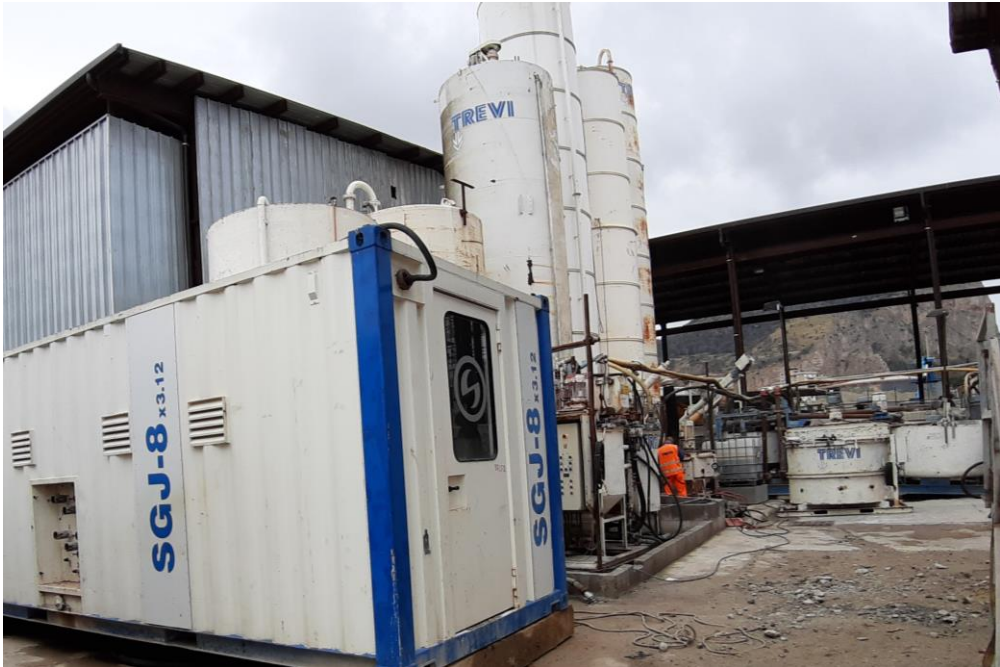
Figure 7-24: Mixing plants installed at Palermo Industrial Port.
