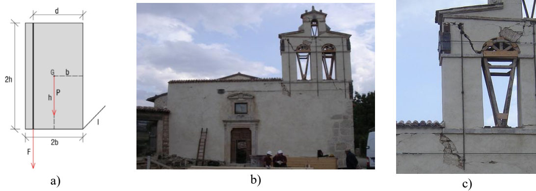
Figure 27: a) Schematic view of the considered bell gable; b-c) Example of a bell gable retrofitted with vertical tie-rods.
