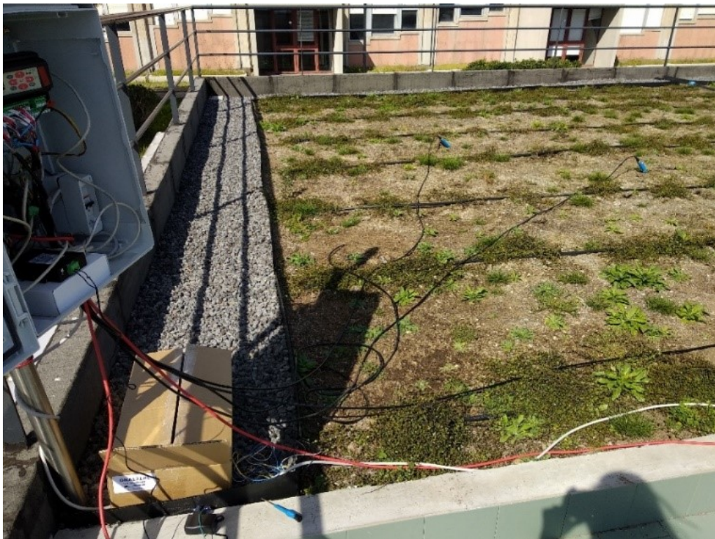
FIGURE 4.9 Master station with 3 TDR sensors.
