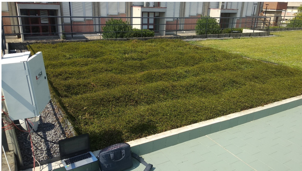
FIGURE 4.7 Master station in the final configuration.
