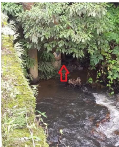
Figure 5 – Inaccessible pipeline due to household waste deposited on the property adjacent to the drainage system
