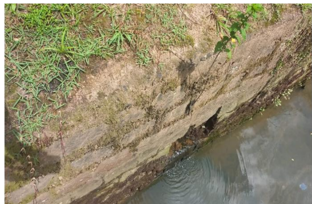
Figure 6 - Water discharge from one of the predefined sampling points during dry weather, possibly indicating groundwater seepage or an illegal sewage connection
