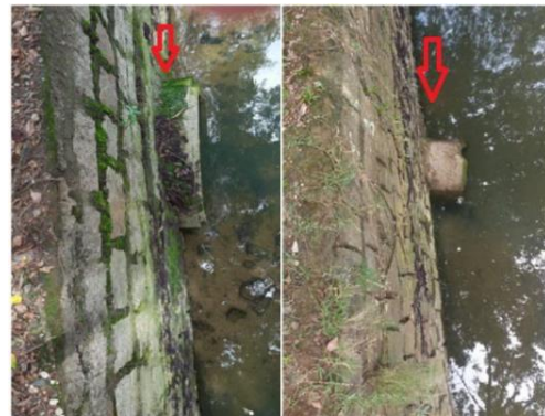
Figure 4 - Limited access due to the drainage pipeline base being close to the riverbed, which could lead to contamination with river water during rainwater sampling
