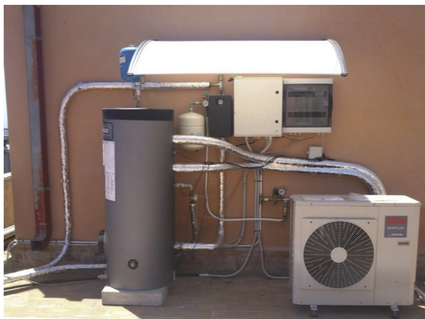
Fig. 3. View of the hydronic section of the PV/T plant.
