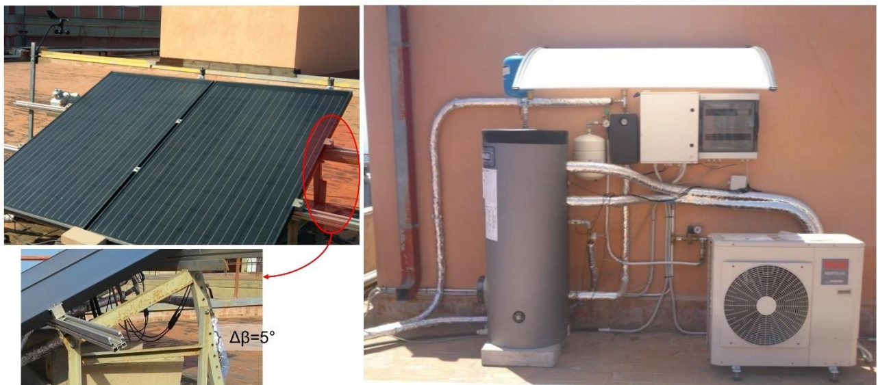
Figure 2.1 – main components of the pilot PV/T system and flexible support structure.
