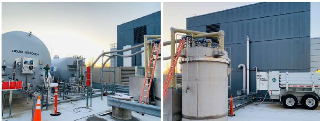
Figure 6. Cryogenic dewars and fill filter.
