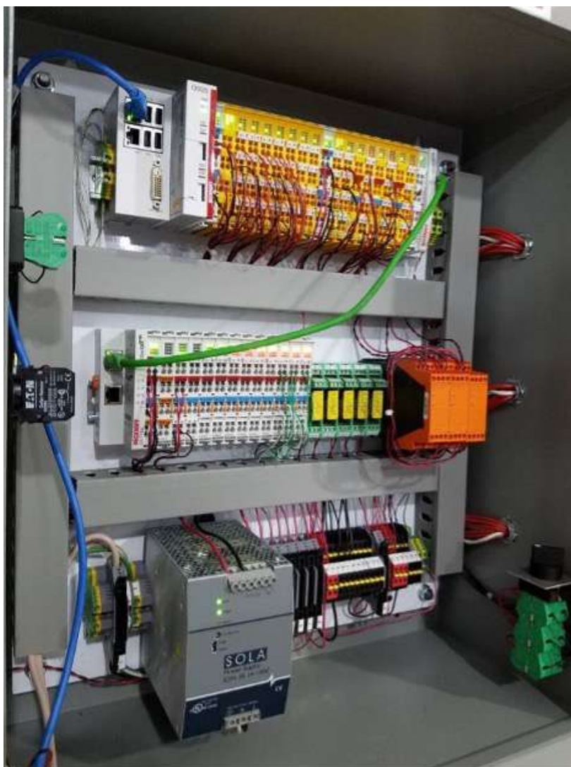
Figure 52. ODH control system enclosure.
