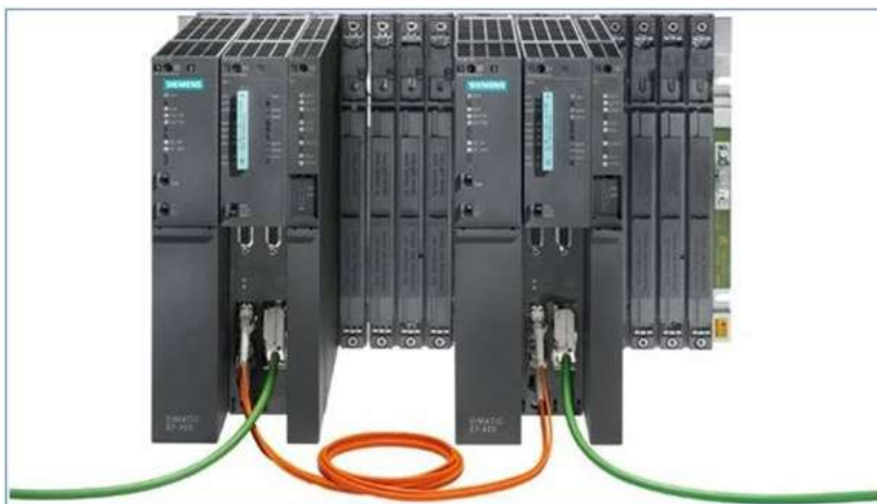
Figure 51. Redundant Siemens S7-400 PLCs.
