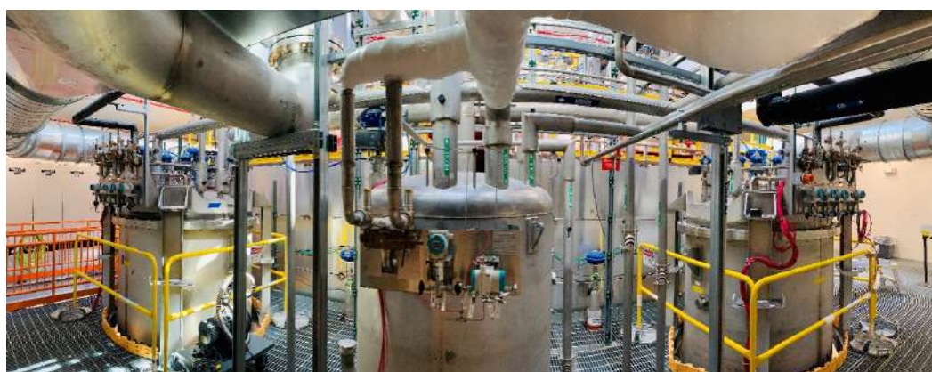
Figure 10. LN 2 phase separator and LAr filter boxes.
