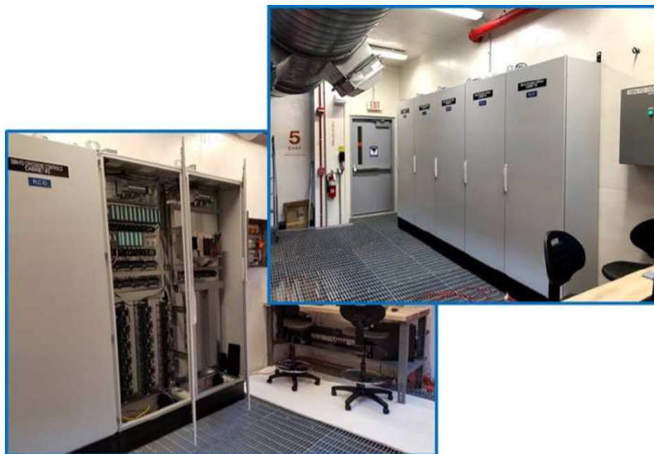
Figure 53. Cryogenic control cabinets.
