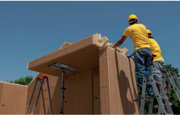
Figure 194/ Assembly of roof panels PACO 120 h250 cm by wooden joints and galvanized steel angular - On-site - University Campus, Catania (CT)
