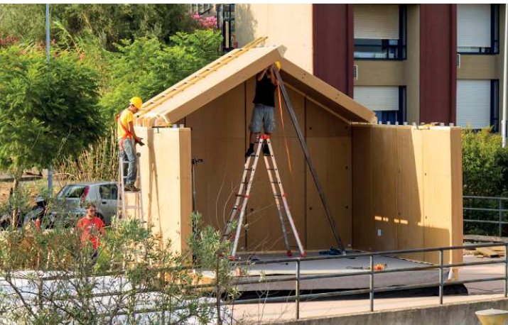
Figure 195/ Assembly of roof panels PACO 120 h250 cm by wooden joints and galvanized steel angular - On-site - University Campus, Catania (CT)
