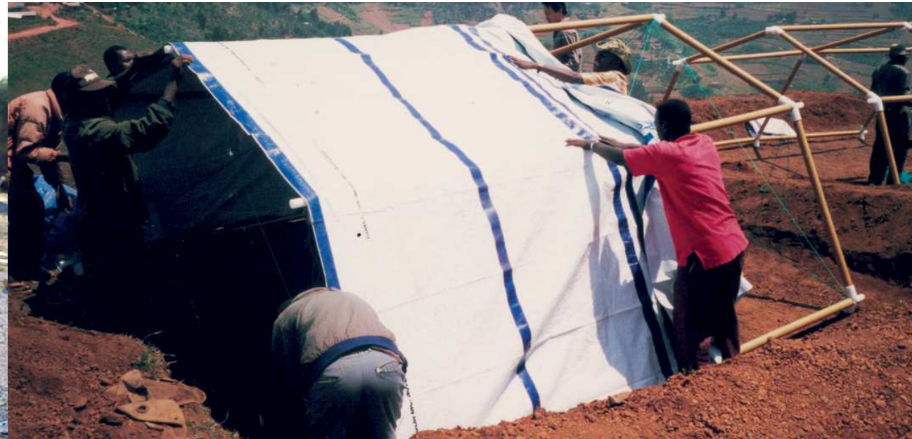
Figure 73 / Paper tubes emergency shelters for the UNHCR at Byumba Refugee Camp in Rwanda, 1999 - © Shigeru Ban Architects - via www.indesignlive.sg
