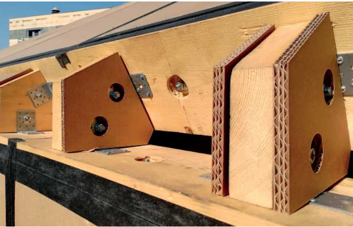
Figure 198 / Preparation of installation of the insulating tube-shaped corrugated cardboard profiles between the wooden joints - On-site - University Campus, Catania (CT)
