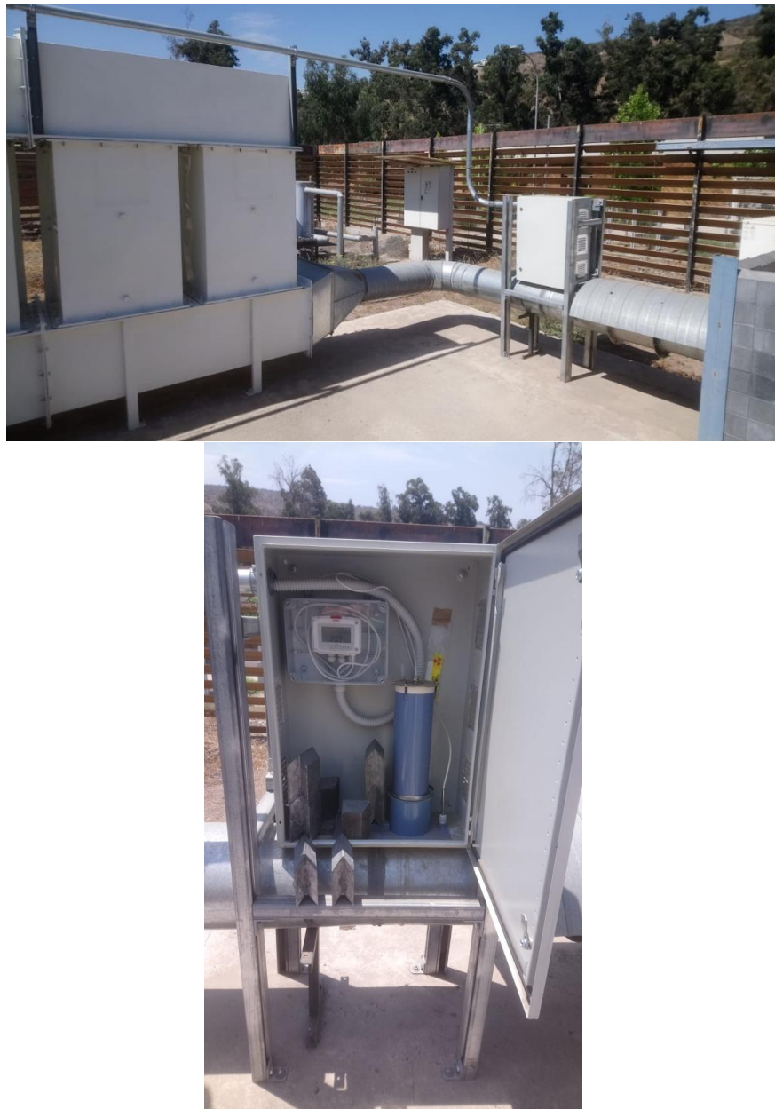
Figure 2.1: Installation of E-STACK-M system for airborne radioactive waste monitoring.
