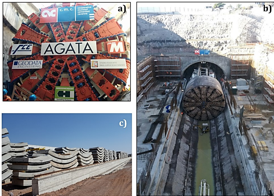
Figure 4.3: TBM utilised along the Nesima-Misterbianco segment: a) front view of the TBM; b) TBM across Fontana station; c) precast concrete segments.
