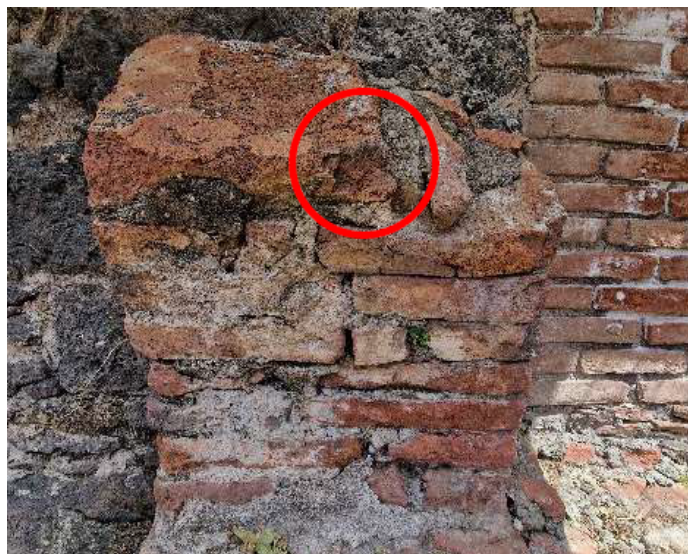
Figure A.16: Sampling point of the Rot_B1_M1 mortar in the praefurnium area of the Terme della Rotonda complex. The image shows the conglomerate wall structure from which the sample was sampled.
