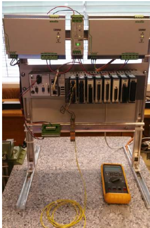
Figure 5.27: The rack is a prototype of the entire Control System; it embeds modules for resistive temperature sensors, pressure sensors, strain gauges, liquid argon level meters, control for heaters. On the upper part a redundant 24 V power supply provides fault tolerant power to the National Instrument controller and modules. Calibration of modules and sensors is ongoing.
