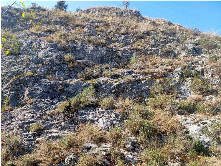
Fig. 4.7. Photograph of the surveyed area on the slope near the viaduct; as can be seen, the rock is heavily fractured and sparsely vegetated.
