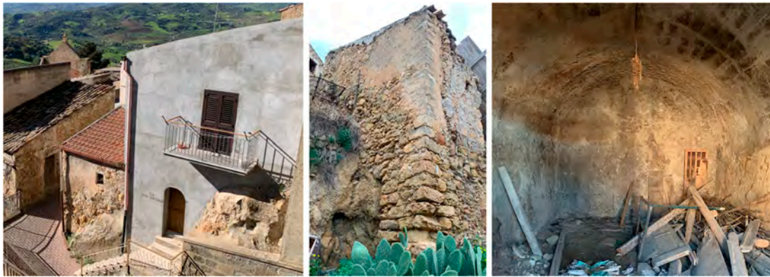
Figure 3. Examples of dwellings built against the rock outcrop. Depending on the ground conditions, the rock outcrop is often an integral part of the elevation walls. Walls are often built directly on natural rock outcrops; similarly, vaults may have a part directly carved into the rock.
