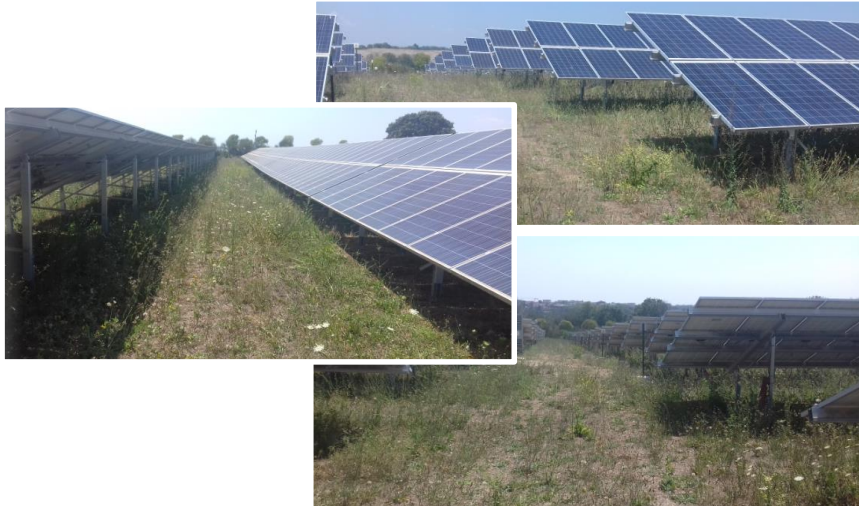
Figure 81. Pictures of the ground-mounted 2 MW PV plant in Central Italy representing the case study 2 of this work
