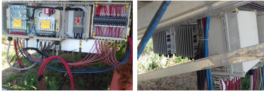
Figure 82. Pictures regarding the assembly of string optimizers. Left: cabling modification at the string box. Right: string optimizers mounted on the back side of the string box
