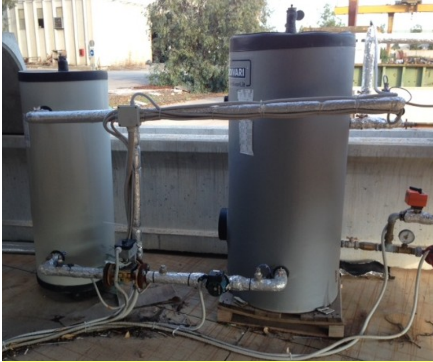
Figure 4. Two main components of the plant: storage tank and boiler
