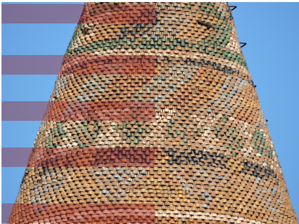
Figure 22. Discontinuities in decorative patterns (highlighted in red) due to the reduction in the number of bricks from one course to the next.
