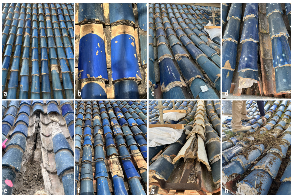
Figure 131. Examples of the main pathologies observed in the roof covering system of the Escuelas Pías church.
