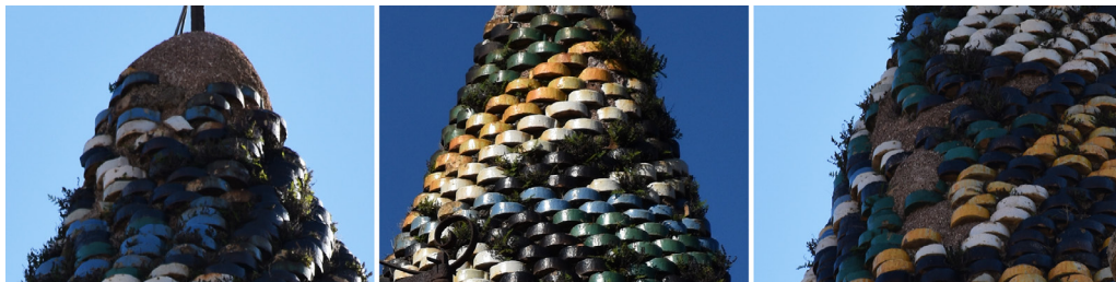
Figure 98. Visible deterioration phenomena: presence of invasive vegetation, glaze erosion, and missing ceramic elements.
