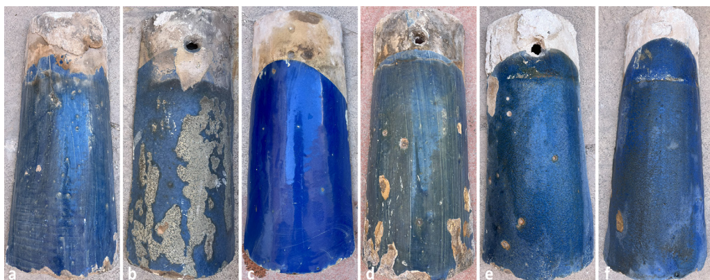
Figure 132. Examples of the main pathologies observed in the tiles of the Escuelas Pías church.
