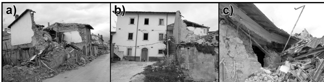
Fig. 2 - Examples of variation of the vulnerability class associated to masonry buildings: a) class B house with external intervention, but the collapse reveals a wall structure typical of vulnerability class A; b) class B edifice (in the background) where the reinforcing prevented significant damage, so the effective vulnerability class becomes C (photo by A. Tertulliani); c) class B house elevated and restored using different materials that create heterogeneity in the structure and overloading; the final behaviour is like a building of vulnerability class A.
