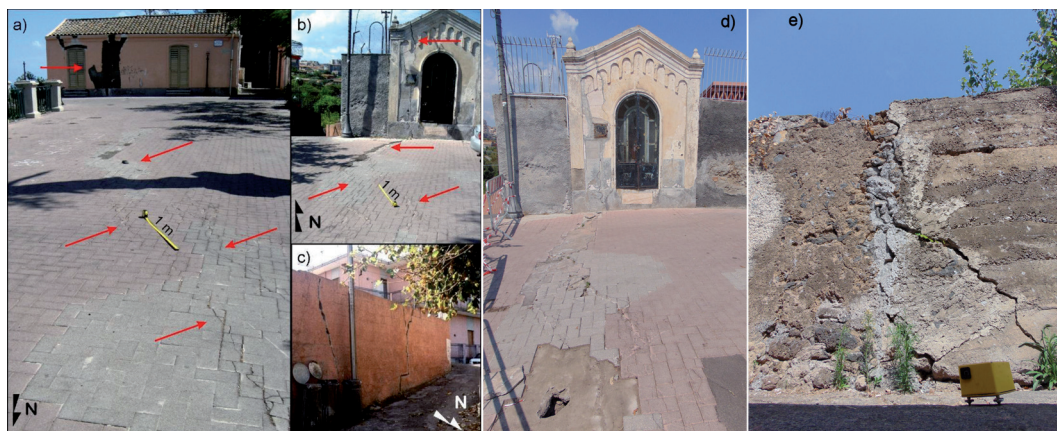
Fig. 1 – Belvedere Place in the S. Caterina village (see Fig. 2 for location), affected by NNW–SSE fractures along: a) the floor and the house; b) the floor and the chapel; c) a wall to the north of the chapel (photographs October 4, 2012, after Barbano et al. , 2014); d) the same chapel and e) via Pianeto (photographs 15 September 2016).
