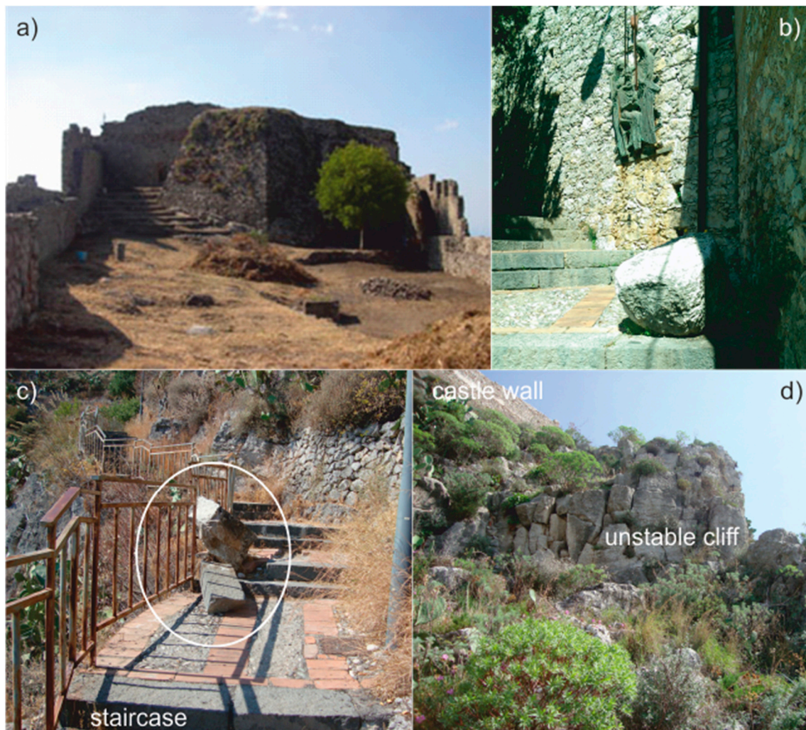
Figure 3. (a) Internal view of the castle; (b) block stopped at a Station of the Cross; (c) block stopped by the banister and damaging the road pavement; (d) loose rock mass.
