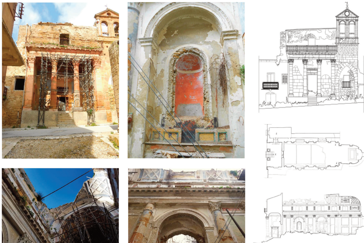
Figure 3. Reconstruction “as and where it was”. Church of Saint Antonio, the Patron Saint.
