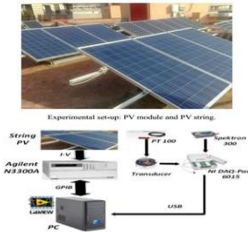
Fig. 2. Renewable energy platform in Catania University-
