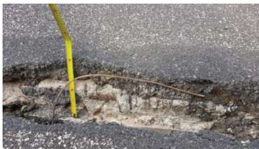
Fig. 7. Bridge Deck, Asphalt pavement and cement concrete deck thickness at the 88 mjoint .
