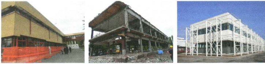
Figure 4. Steps of the seismic retrofit of the Magneti Marelli headquarters in Crevalcore, Italy.
