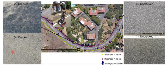
Fig. 2. Selection of pavements in different conditions.
