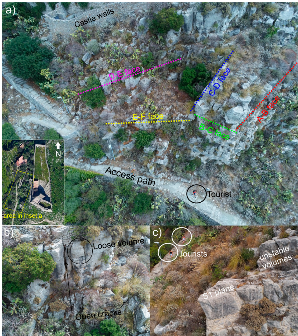
Figure 6. Representative photos from UAV: (a) slope faces with visible loose rock volumes impending over the access path; (b) open cracks isolating rock volumes; (c) a close image of the dip-slope plane enhancing planar sliding over the access path crossed by tourists.
