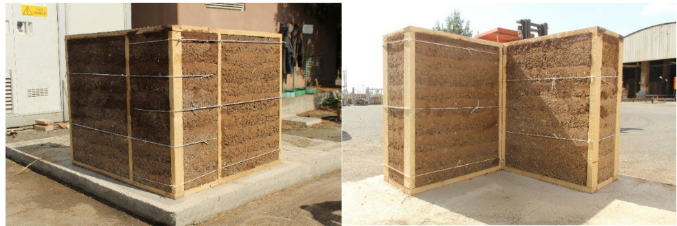
Figure 4. Construction of a prototype wall for the validation of the constructive process: view of the corner from the outside (image on the left) and the inside (image on the right).
