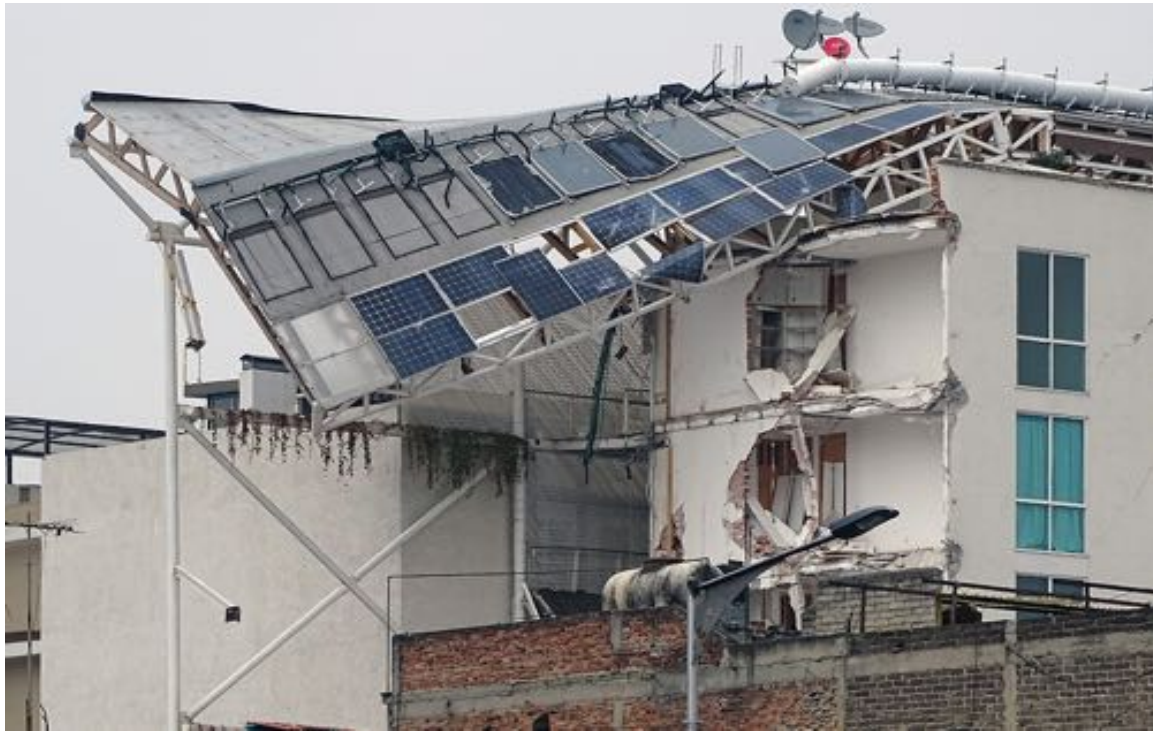
Figure 2. A 7-story building renovated only in terms of energy efficiency, partially collapsed after the earthquake that struck Mexico City in 2017 [9].
