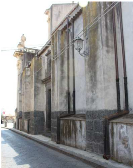
Figure 5. Buttresses placed on the south side of the church of Santa Maria della Catena in Acicatena (photo: A. Lo Faro).
