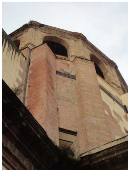
Figure 2. Palermo, Church of SS. Salvatore, hoops placed at the base of the dome.
