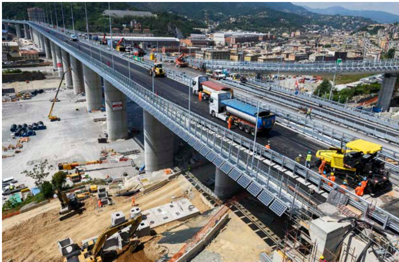
Fig. 1. Laying of the asphalt mixes on the Genova San Giorgio Bridge (July, 2020)
