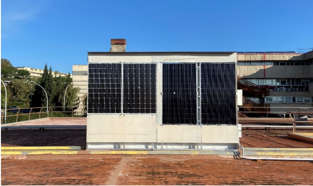
Figure 8 Building ventilated façade with integrated bifacial photovoltaic modules installed at the University of Catania (Italy)
