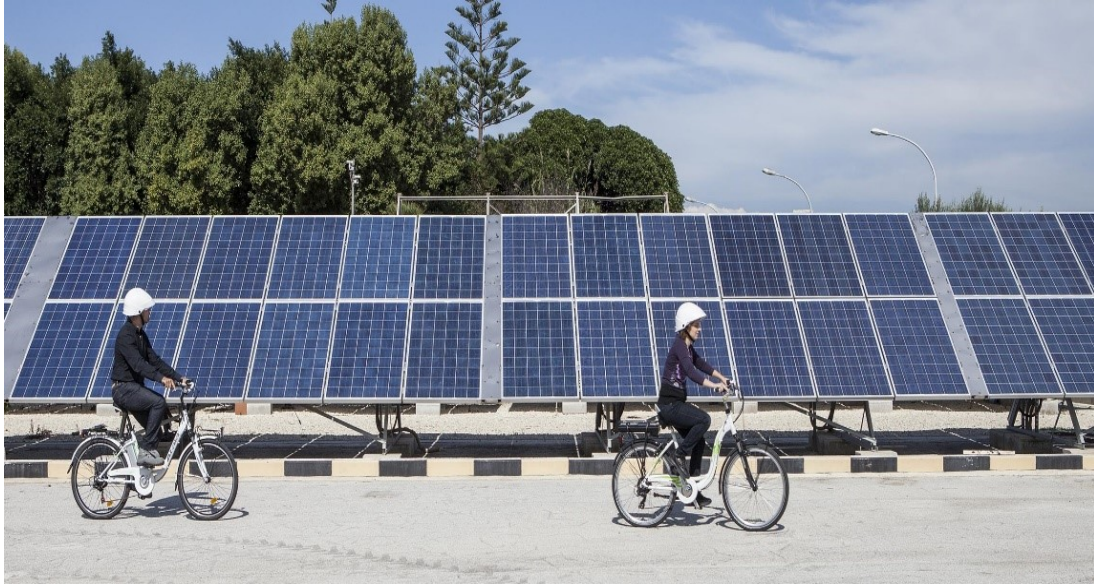
Figure 24 Ground mounted PV plant (GPV)
