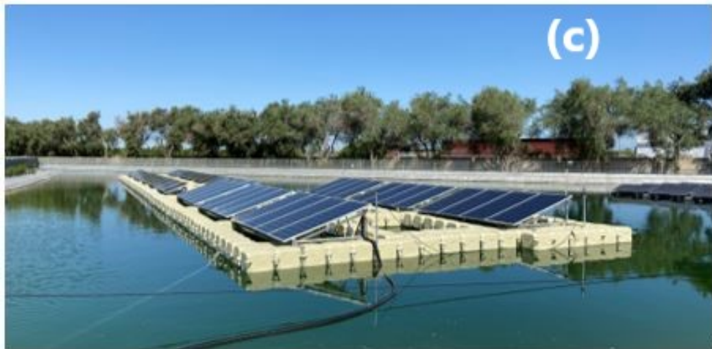
Figure 23. A 6 different solution installed in the lake of EGP
