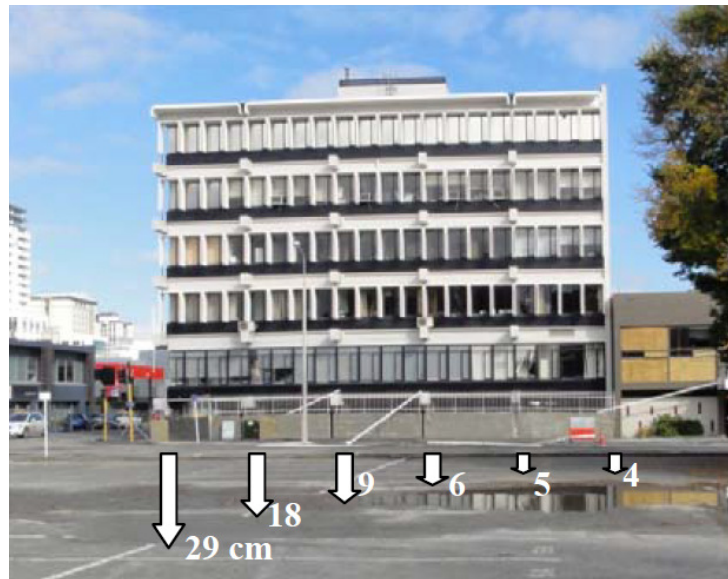
Figure 2.14 Differential settlement of a 6 storey reinforced concrete building in the city of Christchurch (From Cubrinovski, 2014).
