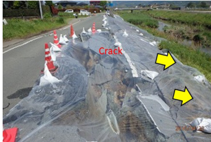
Figure 2.15 Liquefaction-induced damage to levee along Akitsukawa-River (From Kiyota et al., 2017).
