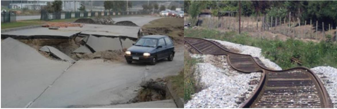
Figure 2.13 Damages to the road infrastructure and railroads system after the 1999 Kocaeli earthquake (From Verdugo and González, 2015).
